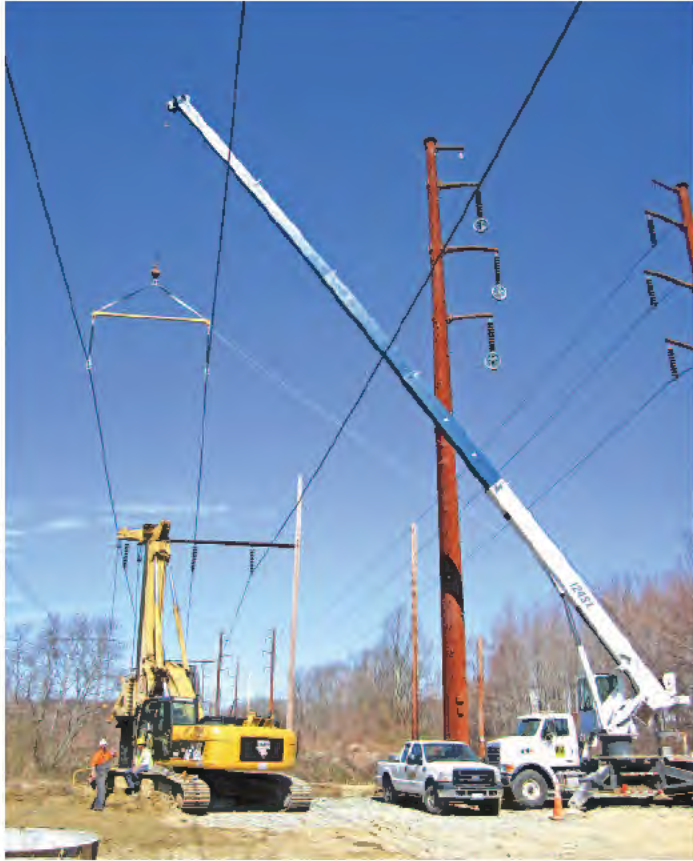
Working under active power lines.
